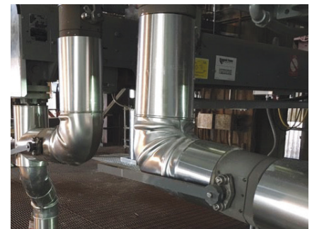
Twenty 2-inch, ASME 600 Class ISOLATOR 2.0 valves were installed in a major utility supplier to isolate steam in the daily operation of soot blowers.
