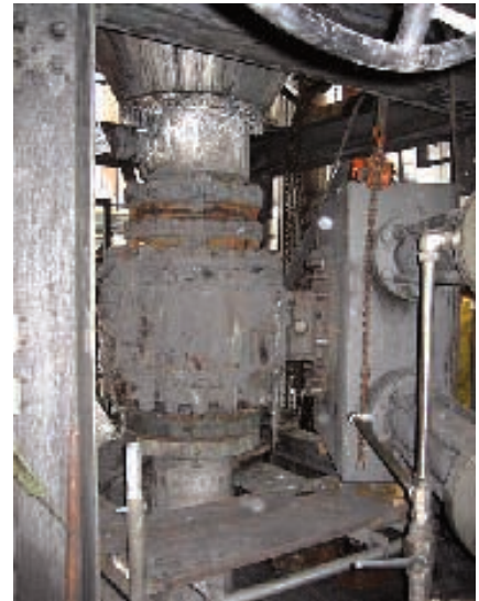
Shown above is the bottom, 16-inch lockhopper valve that endured several years of arduous service, cycling every 15 minutes and discharging erosive slurry.
